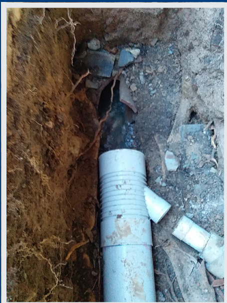
The liner being wound through broken sections and joined with PVC couplers
